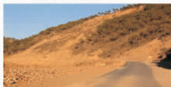
图12 巫溪-巫山公路开挖诱发滑坡 Fig. 12 Landslide triggered by artificial cutting along highway between Wuxi county and Wushen county
