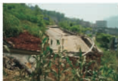
图11 南溪滑坡破坏公路 Fig. 11 Destructive highway in Naxi landslide
